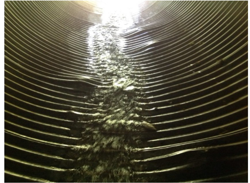
damage to floor
